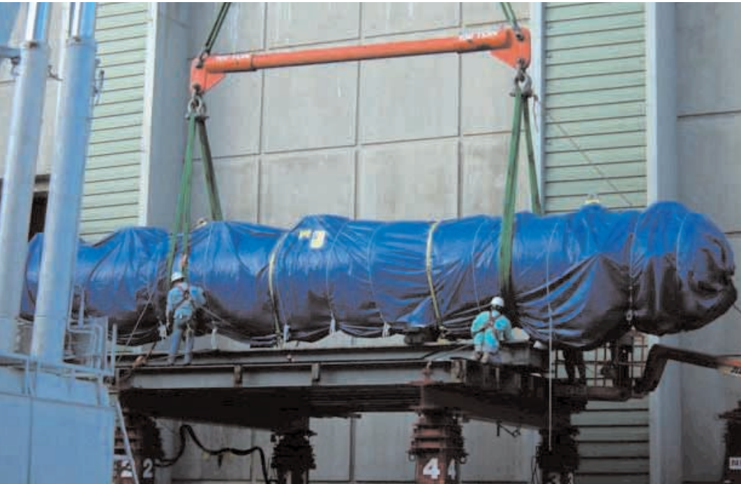
Feedwater heater packaged and ready for transport.
